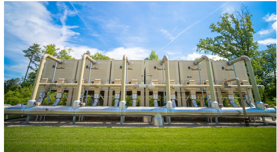
Creative Composite Group: TowerTech cooling tower, NetApp Data Center
