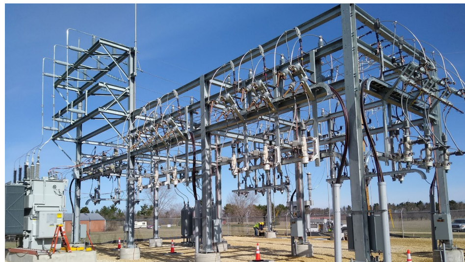
V&S Utilities: substation structure in New Amsterdam, Wisconsin
